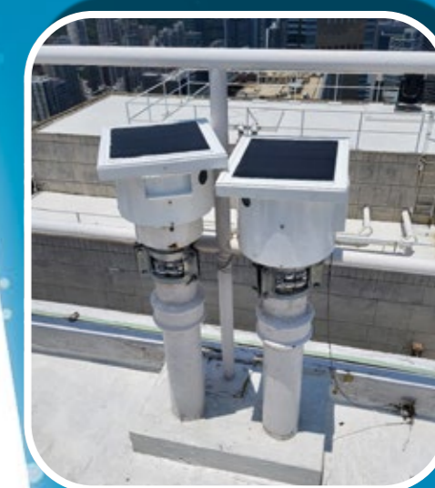
SVP Model III installed at terminal of vent pipe on roof
